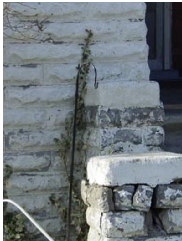
Deteriorated pre-cast concrete foundation
