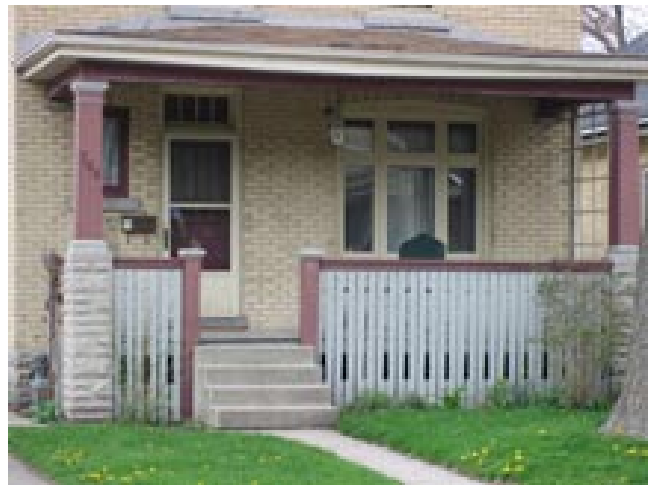
Porch with pre-cast concrete pier and one-piece balusters that extend to ground
