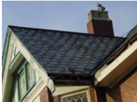
Weathered fascia with portions of soffit missing
