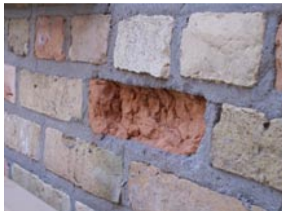
Example of brick spalling, where exterior layers have crumbled off centre brick
