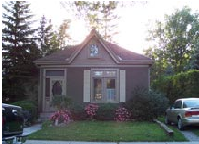
Well executed stucco replacement with respect to colour, texture and retention of details
