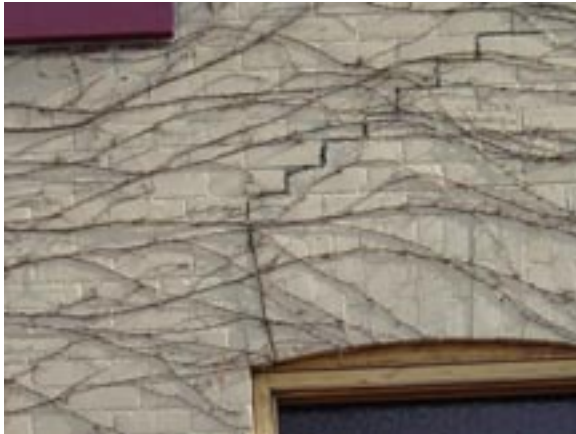
Minor settlement and cracking in brickwork
