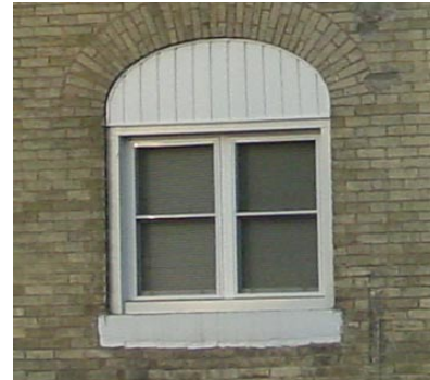
Avoid removal of stained glass window features
