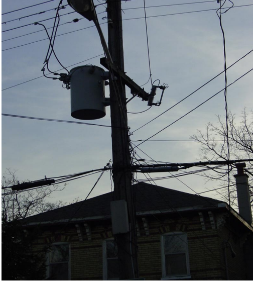
Utility pole at 485 English
