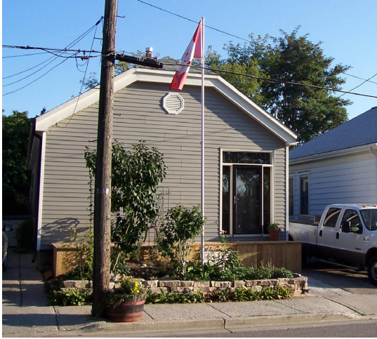
Inappropriate use of vinyl siding, cladding over windows and details
