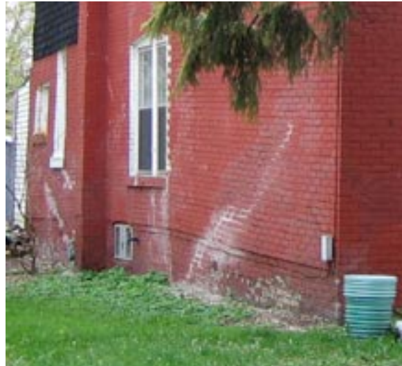
Serious brick settlement and instability. White deposits indicate efflorescence
